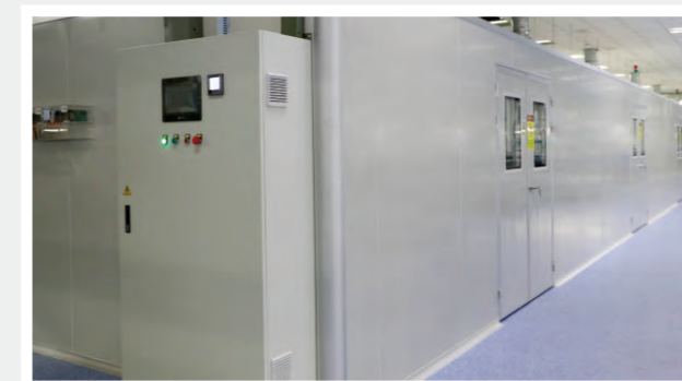
High temperature and load aging room
